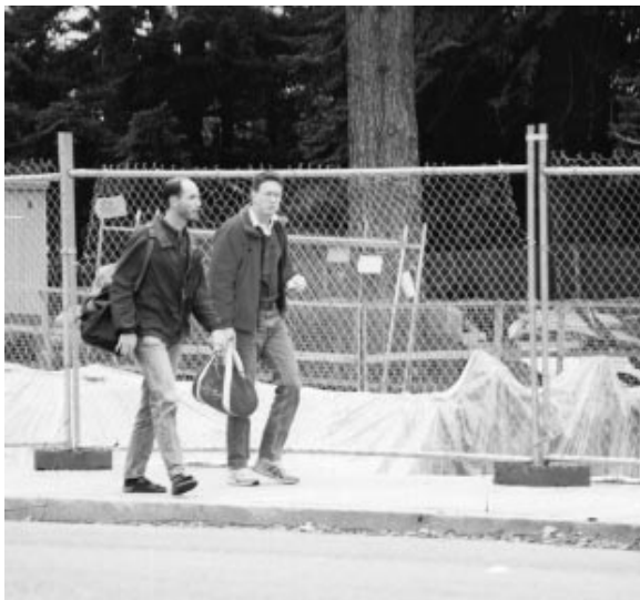
Fencing used to secure a work area supported by blocks needs to be positioned to avoid creating obstacles or tripping hazards for pedestrians.
